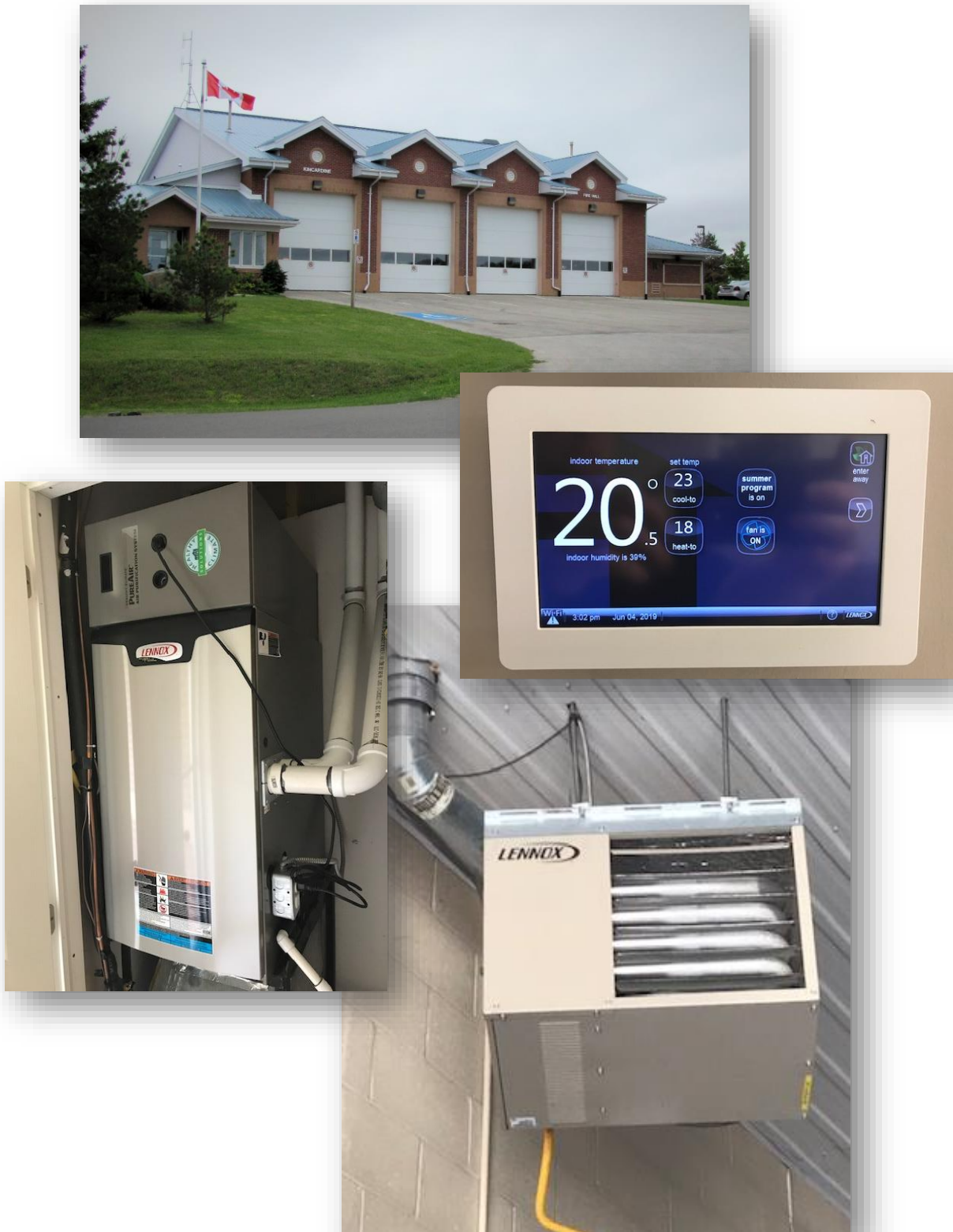
Figure 2: New high efficiency ceiling mounted furnaces, instantaneous water heaters, programmable thermostats and LED lighting fixtures at the Kincardine Fire Hall
