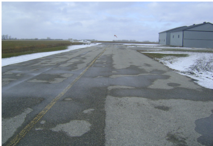
Typical Pavement Conditions on Taxi C
