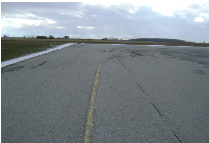
Typical Pavement Conditions on Taxi A
