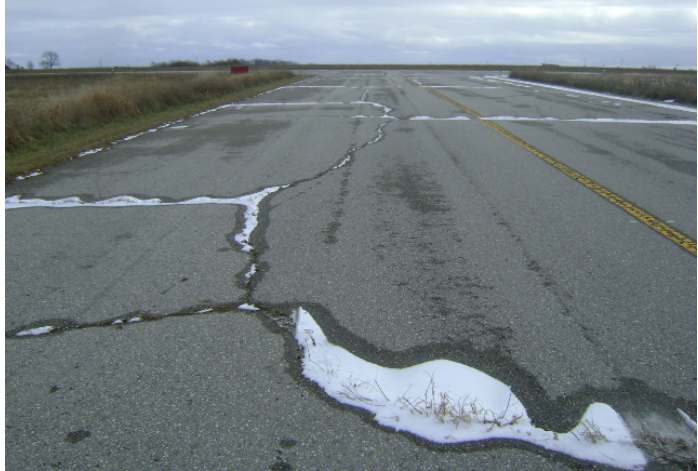
Typical Pavement Conditions on Taxi D
