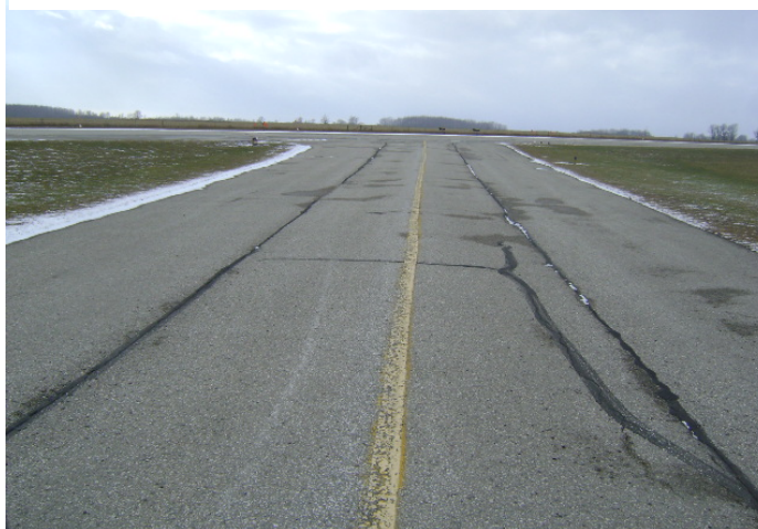
Typical Pavement Conditions on Taxi B
