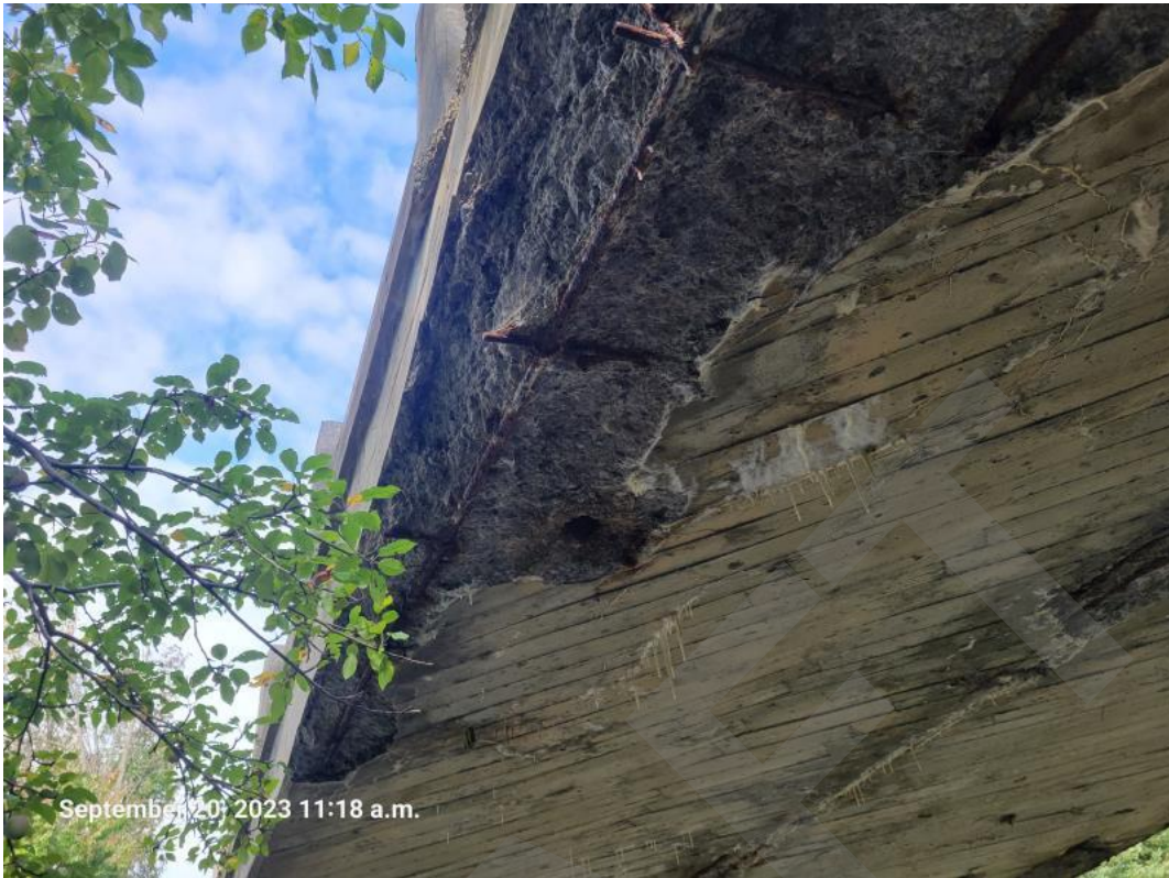
9-Deck Spall at Southeast Drain
