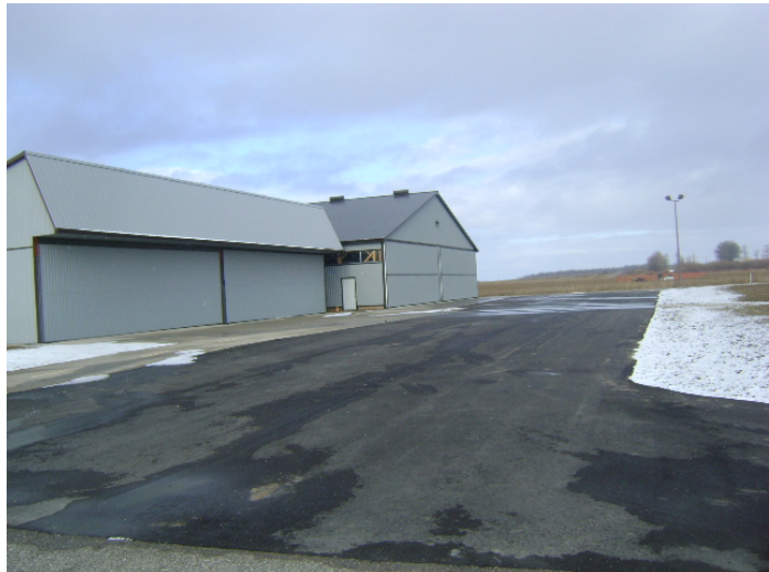
Typical Pavement Conditions on Taxilane System
