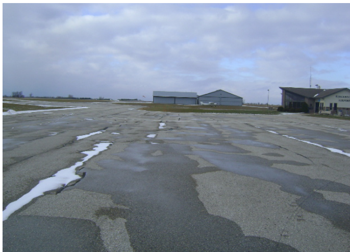
Typical Pavement Conditions on Apron I
