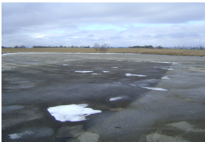
Typical Pavement Conditions on Apron II
